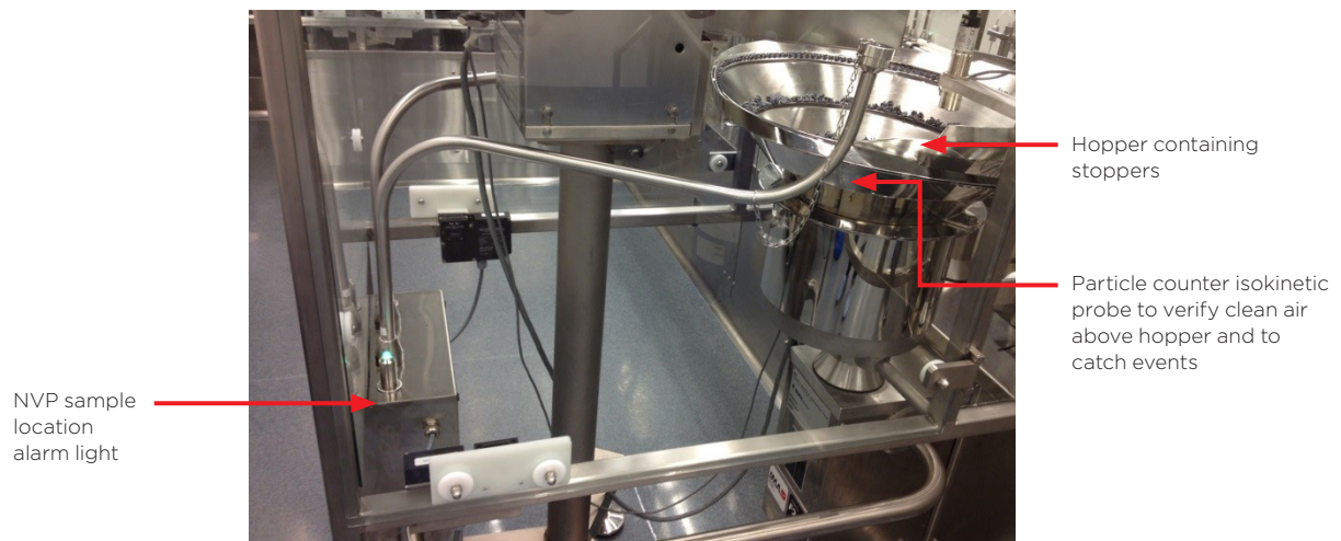
Figure 1. NVP monitored Hopper inside clear isolation barrier
